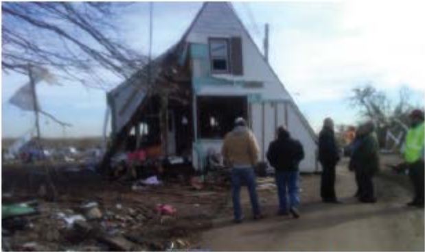
A house in Oakwood Beach that was pushed into the street by storm surge.
