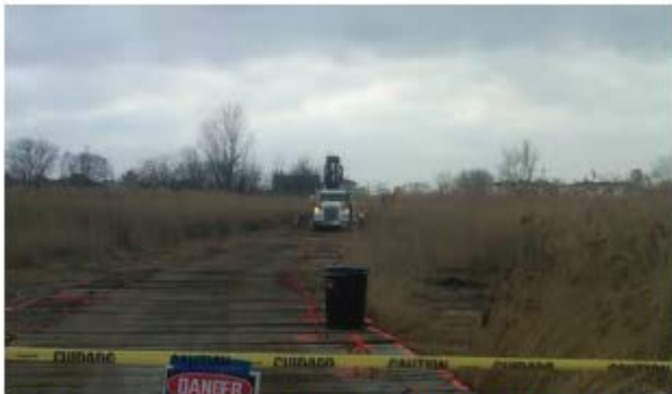
Protective mats were laid in the Oakwood Beach wetland during debris removal.
